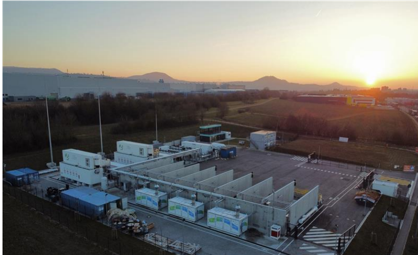
Schwäbisch Gmünd, 10 MW bulk site (Bade-Wurtemberg, Germany)
