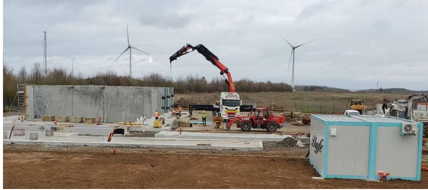
Croixrault 5 MW bulk site, Hauts-de-France, France
