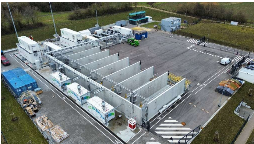
Schwäbisch Gmünd 10 MW bulk site, Bade-Wurtemberg, Germany
